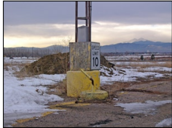
Site improvements in and around the dog track parking lot showed signs of deterioration.
