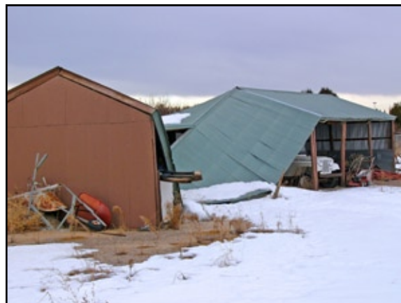
An ancillary structure at the dog track had partially collapsed.
