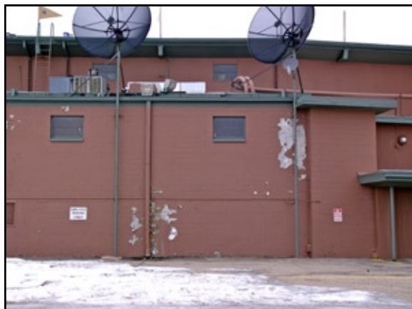
Both the dog kennel and the dog track showed signs of exterior deterioration.
